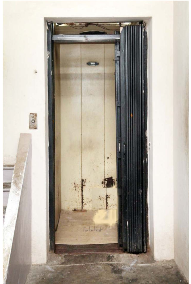
Lift – 2 in Hostel
