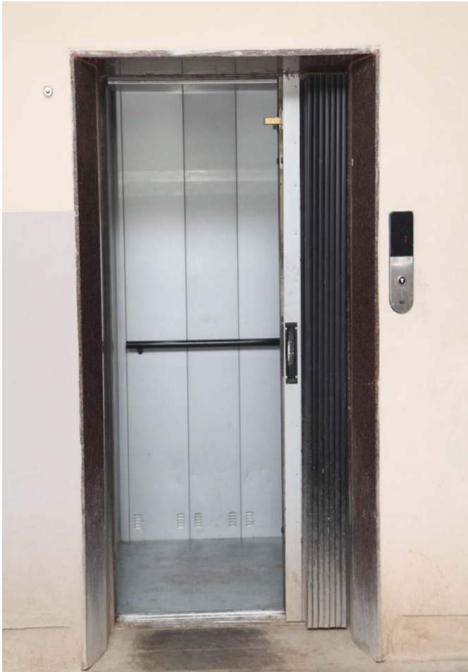
Lift – 1 in Hostel
